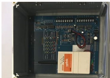
Sewer Lift Station Monitoring System
