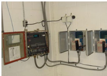
Radio tower light monitoring system
