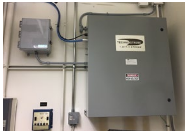
Backup generator monitoring system
